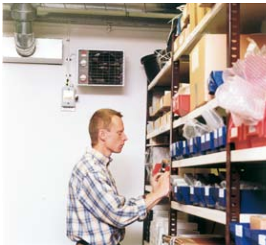
Premises that are only used occasionally can be quickly heated when required with a fan heater.
